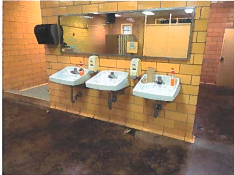
Sink/shower area showing raised ledge that needs to be removed
